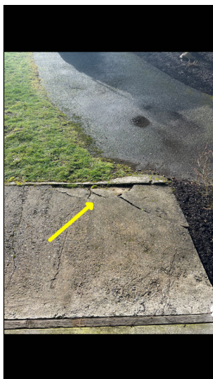
Cracked apron in front of garage.
