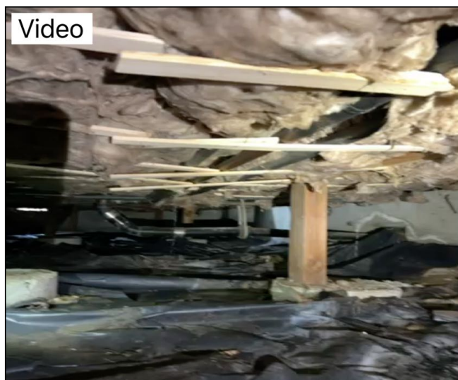
Active leaking from kitchen sink, drain line.
