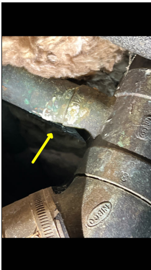
Leak from kitchen sink that ties into waistline.
