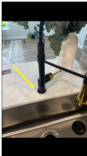
Faucet loose at base.
