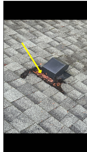
Another poor repair made on roof flashing.
