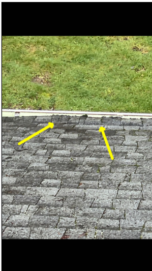
Curling shingles at the low edge of the roof.
