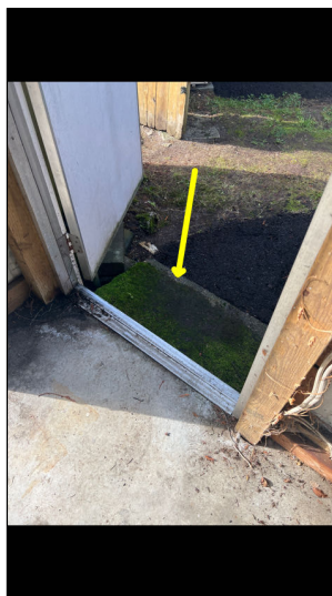
Moss covered apron by service door.
