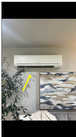
Mini split located in living room.
