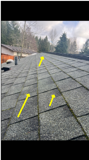
Moss on roof
