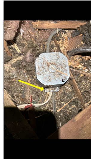
Example of properly clamped wires.
