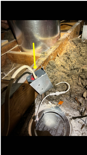
Wire not clamped to box.
