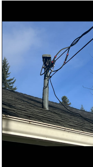
Service drop in good shape.
