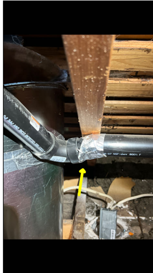
Poor connection in vent line. (Should be glued)
