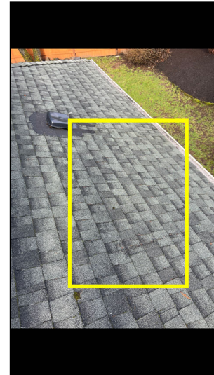
Area of shingle damage.
