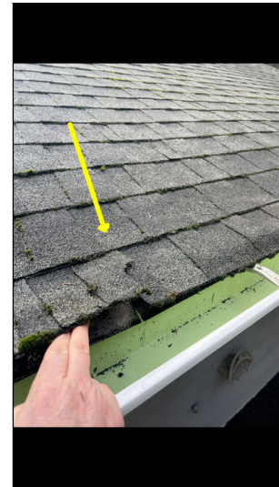
Broken shingle on edge of roof.
