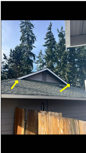
Trim touching roof edge.
