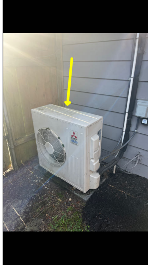
Heat pump AC unit.
