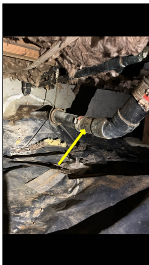
Negative grade on waste line.
