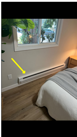
Electric wall heat.
