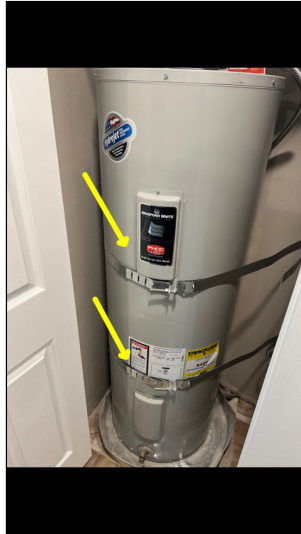
Water heater strapped.
