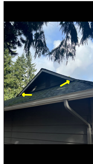
Trim touching roof edge.
