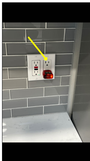
Outlet not GFCI protected.
