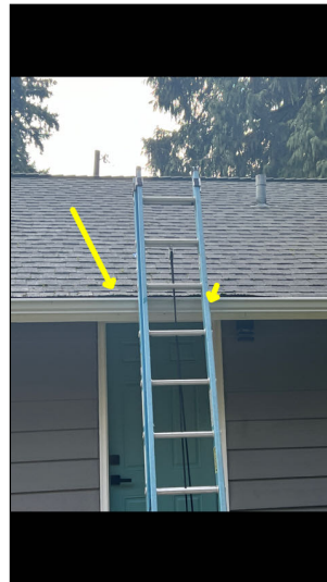
Area of damaged shingles.
