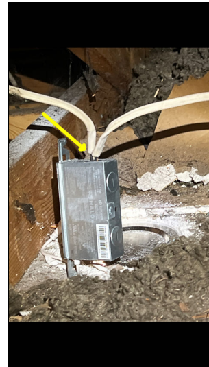
Wire not clamped into box.
