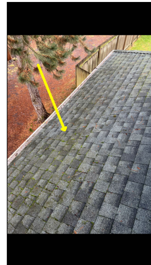
Moss on roof.
