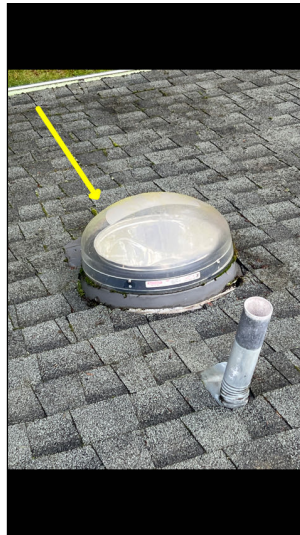
Solar tube skylight
