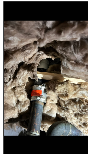
Questionable repair made to bathtub drain line.
