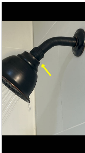
Shower head leaks.
