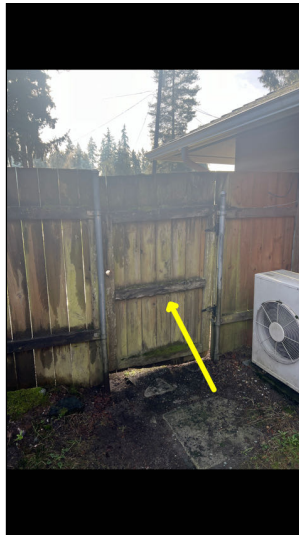
Poorly functioning gate.
