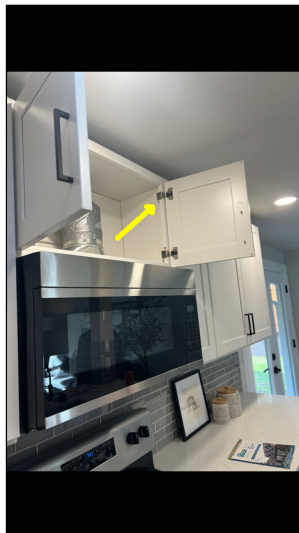
Loose top hing just needs to be tightened.
