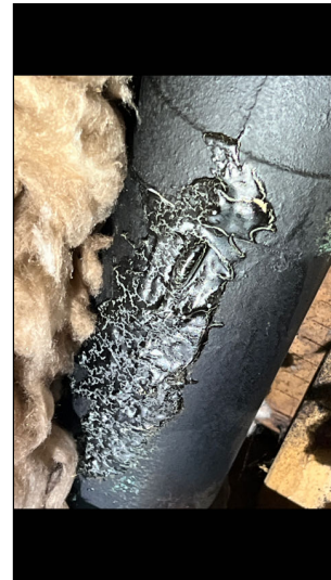
Questionable repair drain line from toilet.
