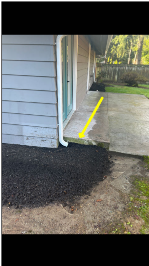
Recommend splash Block under downspout.
