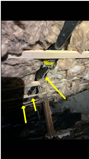
Waistline for kitchen sink leaks in several spots needs to be replaced.
