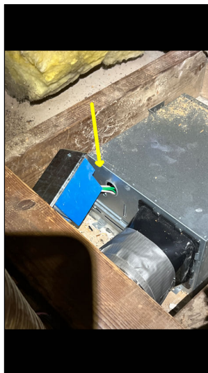
Electrical for exhaust fan and bathroom is not properly secured.
