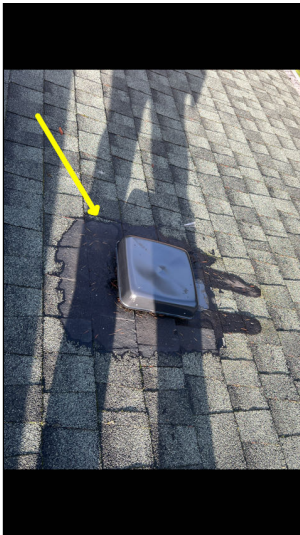
Poor repair job.
